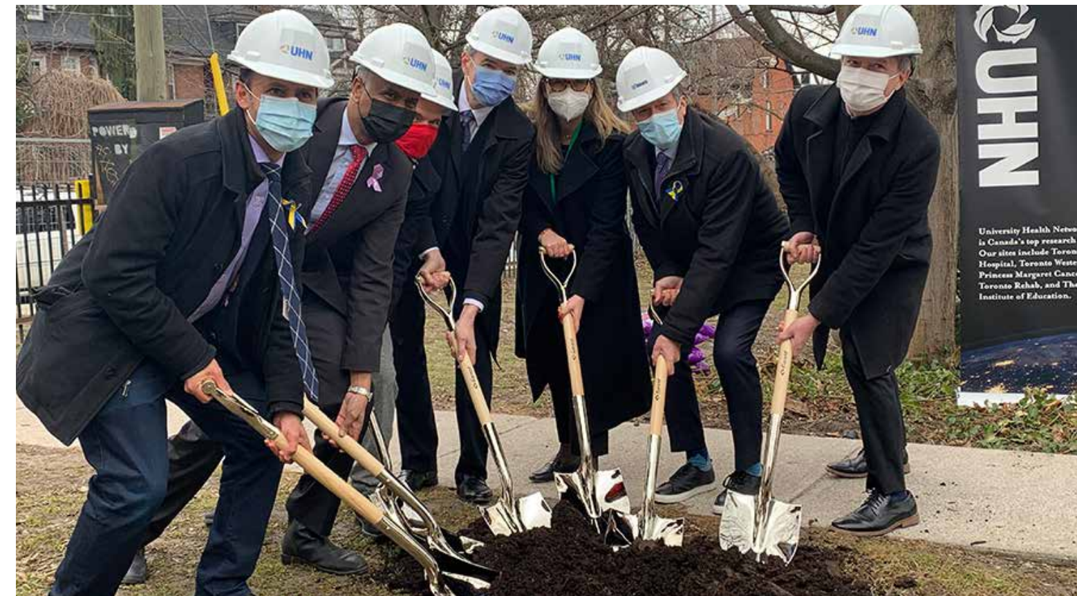
Helping kick off the construction of the Social Medicine Supportive Housing project in Parkdale were: (L to R) Arif Virani, MP for Parkdale-High Park, the Honourable Ahmed Hussen, Minister of Housing and Diversity and Inclusion, Daniele Zanotti, President and CEO, United Way Greater Toronto, Dr. Kevin Smith, President & CEO of UHN, Toronto Deputy Mayor Ana Bailao, Toronto Mayor John Tory and Gord Perks, City Councillor, Ward 4, Parkdale-High Park. (Photo: UHN)
